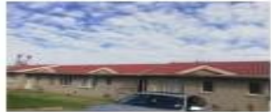
Block of units from 1-4 25m front gutters and Fischer board 20m back gutters and Fischer board
