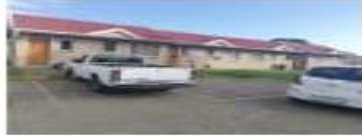
Block of units from 21-24 25m front gutters and Fischer board 20m gutters back and Fischer board
