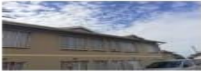
Block of units from 110-112 15m front gutters and Fischer board Back 18m gutters and Fischer board
