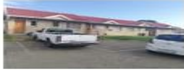
Block of units from 21-24 25m front gutters and Fischer board 20m back gutters and Fischer board
