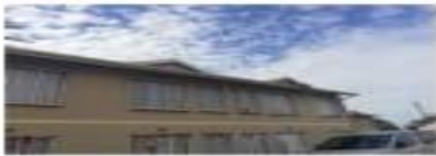
Block of units from 110-112 18m front gutters and Fischer board back 18m gutters and Fischer board
