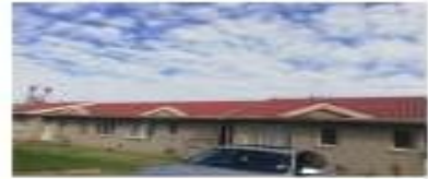
Block of units from 1-4 25m front gutters and Fischer board 20m back gutters and Fischer board
