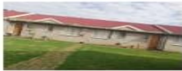
Block of units from 27-28 25m front gutters and Fischer board 20m back gutters and Fischer board
